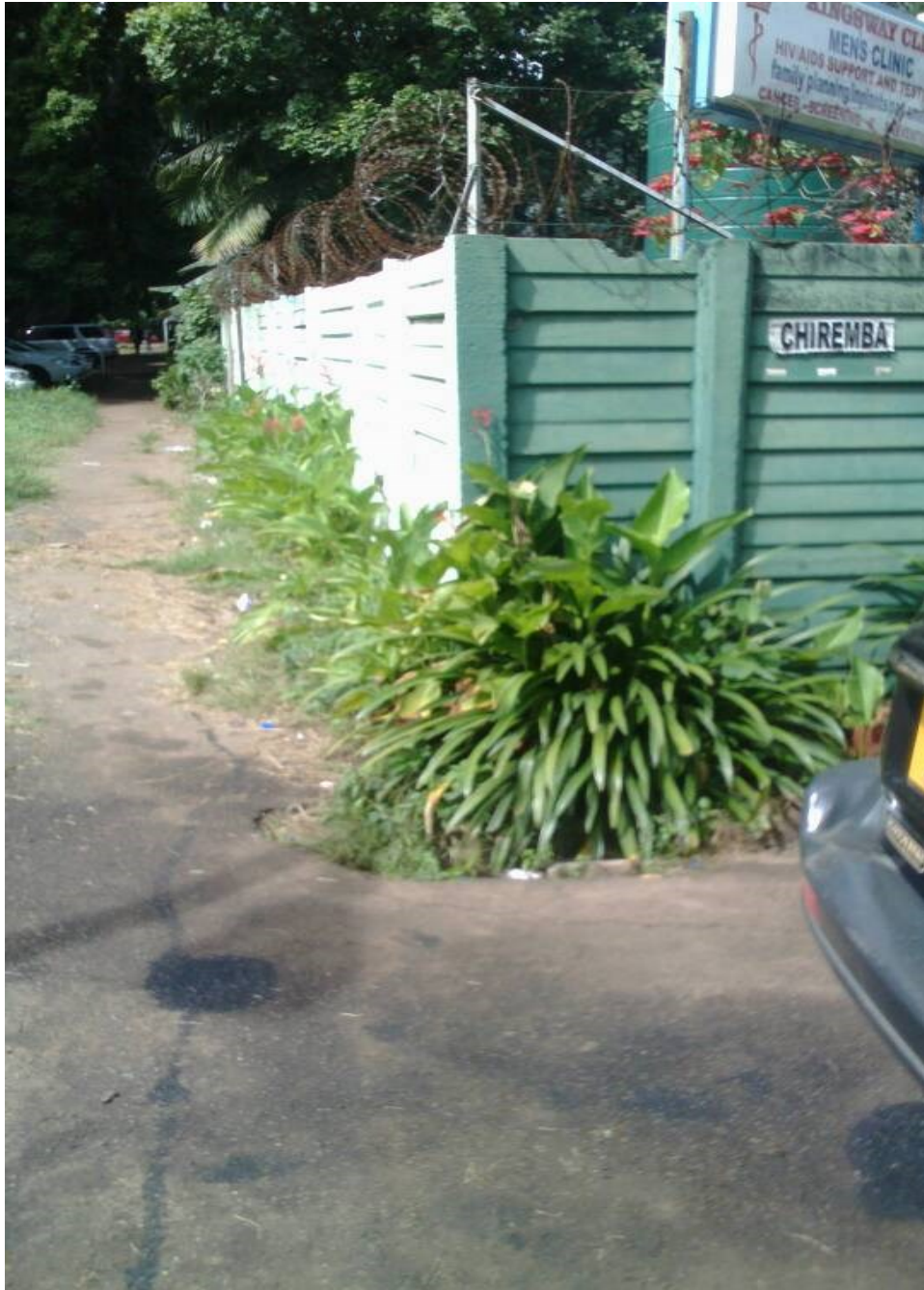
Figure 6: Photograph of a dangerous open drain situated about 100m from the Braille Library in Harare
