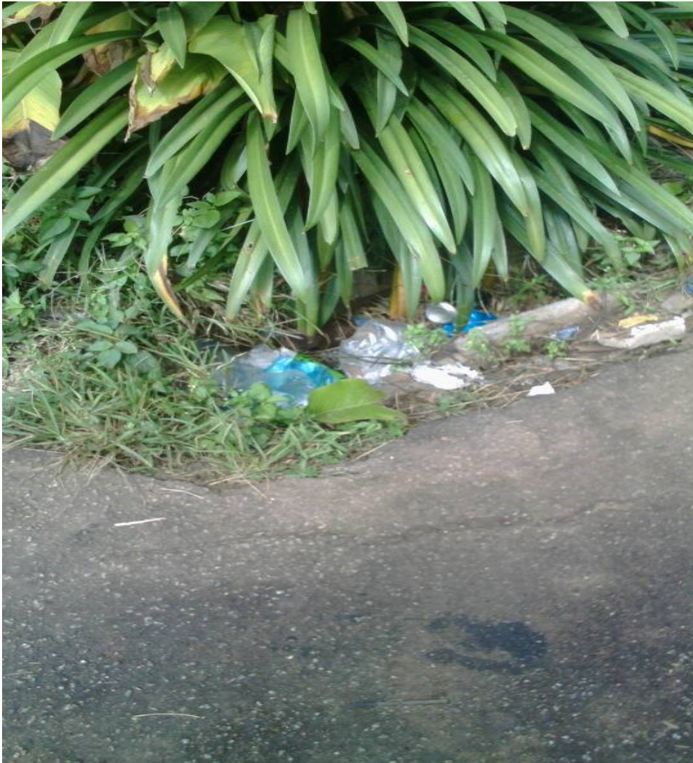
Figure 7: Close-up photograph of the dangerous open drain shown in Figure 6 showing the rubbish which has accumulated in it
