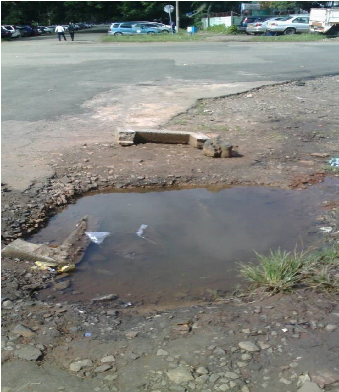
Figure 8: Photograph of a dangerous pothole at a traffic intersection about 50 metres from the Braille Library in Harare
