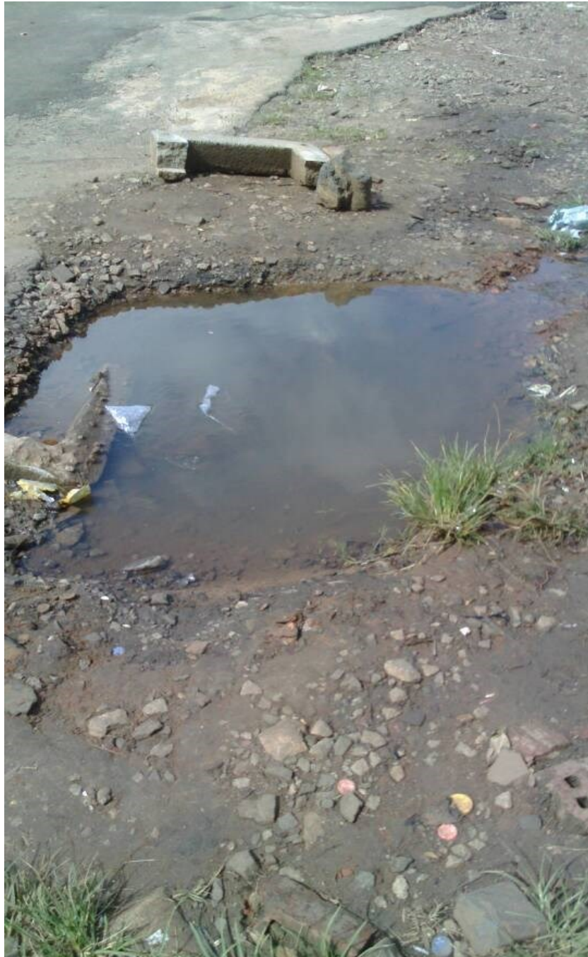
Figure 9: Close-up photograph of the dangerous pothole shown in Figure 8
