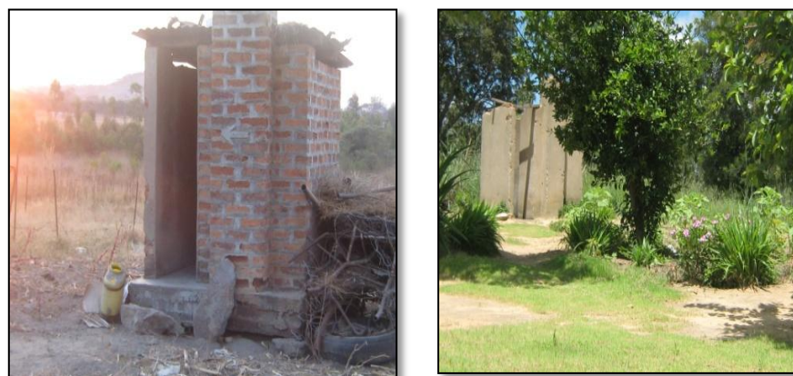
Figure 13: Pit toilets built at Saga Farm, prior to and post to FTLRRP
