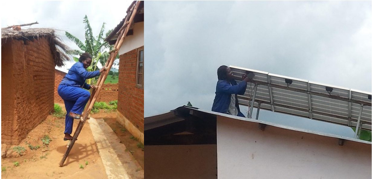
Figure 9: Photographs of Mary caught in action climbing a ladder to a roof (left) where she installs a solar panel (right)
