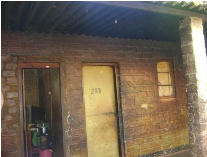
Figure 0-2: the outside and inside part of a block of rooms in Ingezi turned sooty because of wood fuel.
