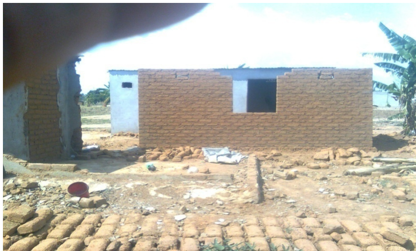
Figure 4: Photograph of a typical house in EPWORTH built for the visually impaired from substandard materials
